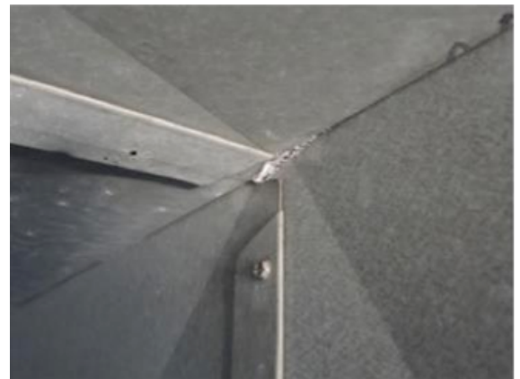
The sealant doesn’t coat the duct interior but accumulates primarily in and around the leaks.
