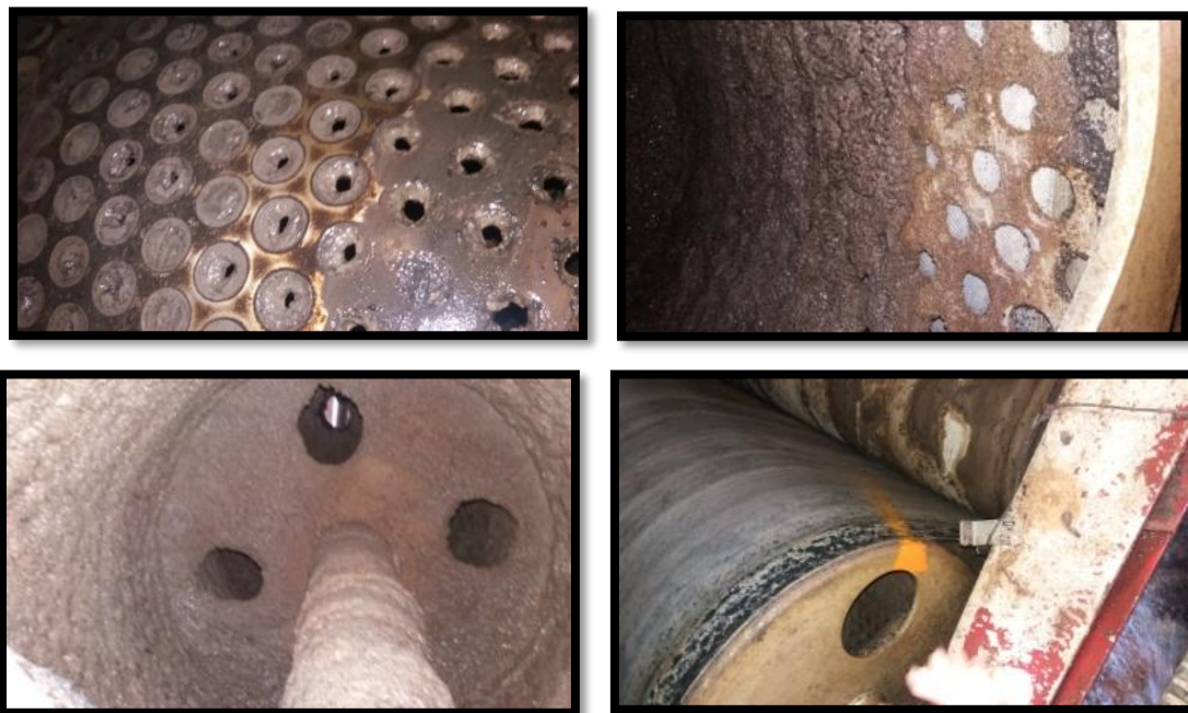
Figure 4: Baseline condition on 7 th September 2017 before HydroFLOW was activated
